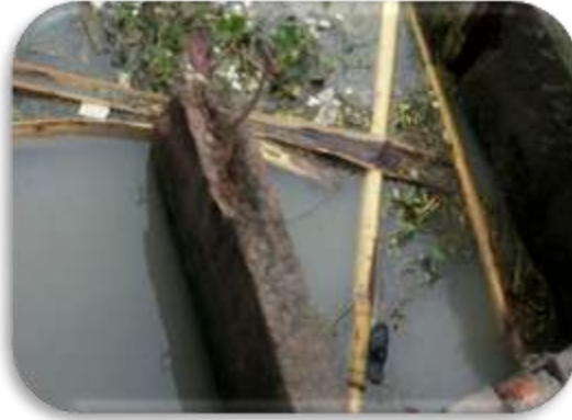
Photo: Damaged gate near Mathabanga in front of Rupsha river
