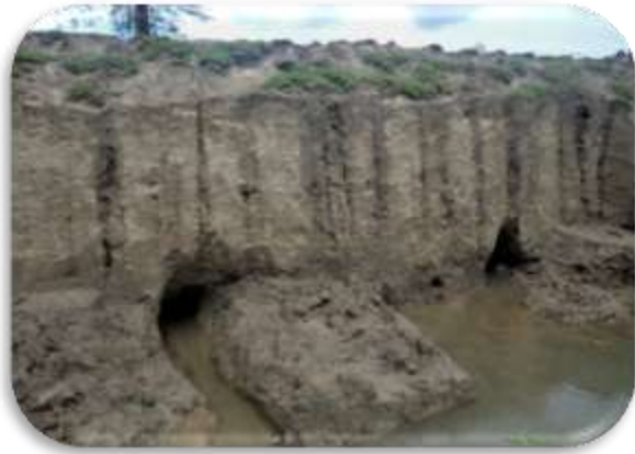
Photo: Saline water easily comes into this damaged embankment in Kasiadanga
