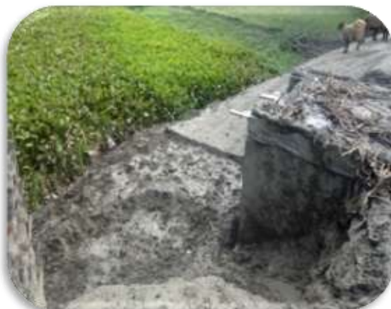
Picture: Gate is blocked in Kasiardanga
